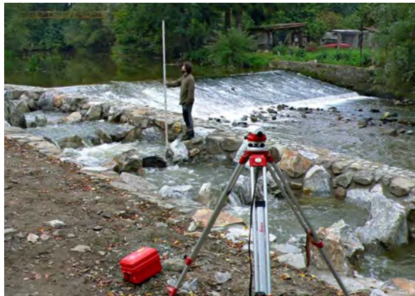
Fig. 7. Fish passage at the weir (upper part of the adjustment) at the old ice stadium in the chateau park, conceived as a concrete channel with lateral boulder steps. NCA workers are levelling the pools in the passage in order to judge the evenness of the fall between the lateral boulder steps. (T. Just)
