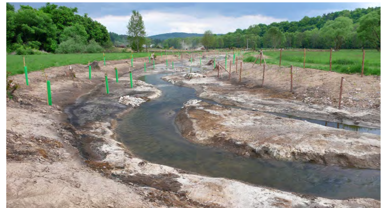
Fig. 1. Revitalised streambed of Loděnický potok stream near Nenačovice, Beroun region, after finishing construction and tree planting, 2015. Activity by Povodí Vltavy, s.p., financed from the Operational Programme Environment. (T. Just)
