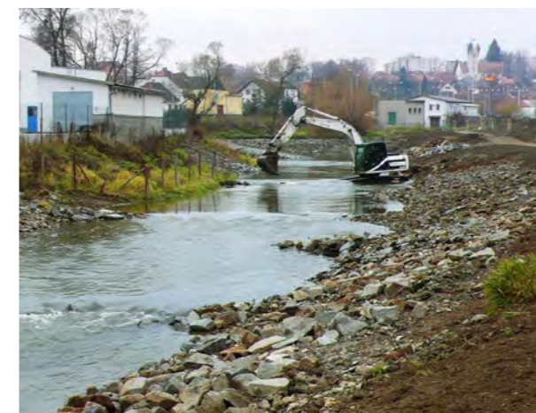
Fig. 3. Blanice at lower outskirts of Vlašim during revitalisation. After removing nutrient-rich soil from the banks and opening up the riverbed, a relatively near-natural riverbed was shaped and then stabilised and diversified with bottom stone strips, spurs and stone riprap structures. (T. Just)
