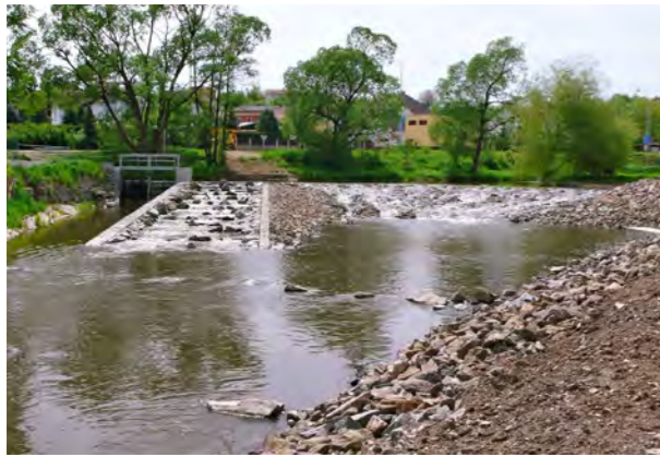
Fig. 6. Weir at Kyselý Laundry after reconstruction. Here, the lower facial side of the weir was filled up to create a stone platform, and a fish passage was built. The passage is made up of a concrete channel with lateral boulder steps. (T. Just)
